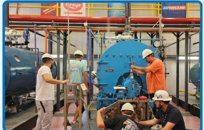
Boiler operation maintenance
